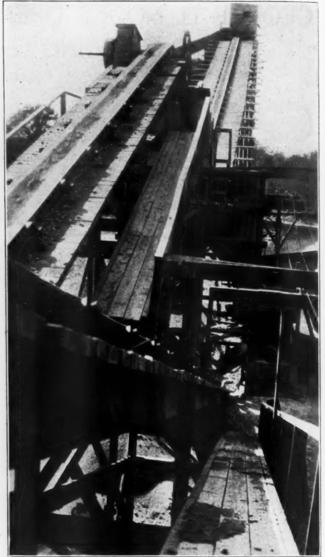
Conveyors to Scalping Screens and from There to Sizing Screens
